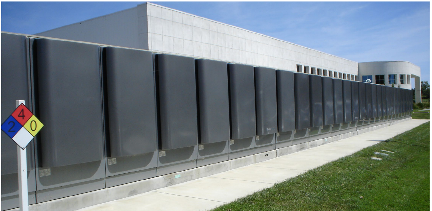
On-site fuel cells at our San Jose, CA, U.S. facility.
