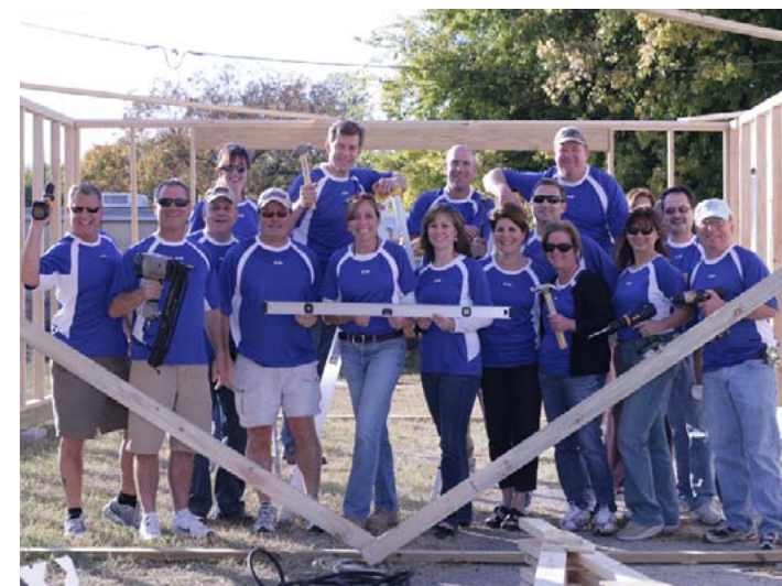
BD associates helped transform an aging elementary school into a community center in San Antonio, Texas, USA.
